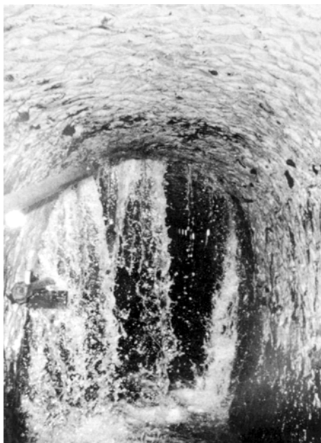
Groundwater flowing from a fracture in the Chalk into a tunnel (or adit) driven from a well in the Lee Valley.
